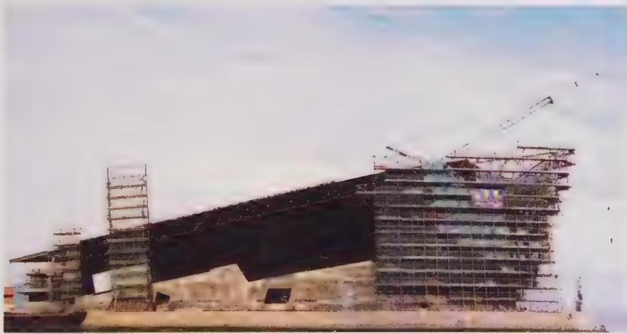
Black waterproof layer of cladding system prior to erection of marine-grade aluminium panels.
