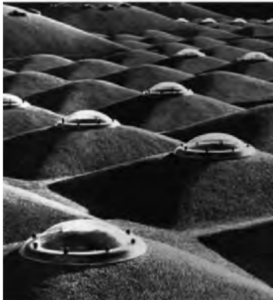
6. (below) The roofscape of small domes, some with central rooflights. This dictated a small scale, appropriate to children.
