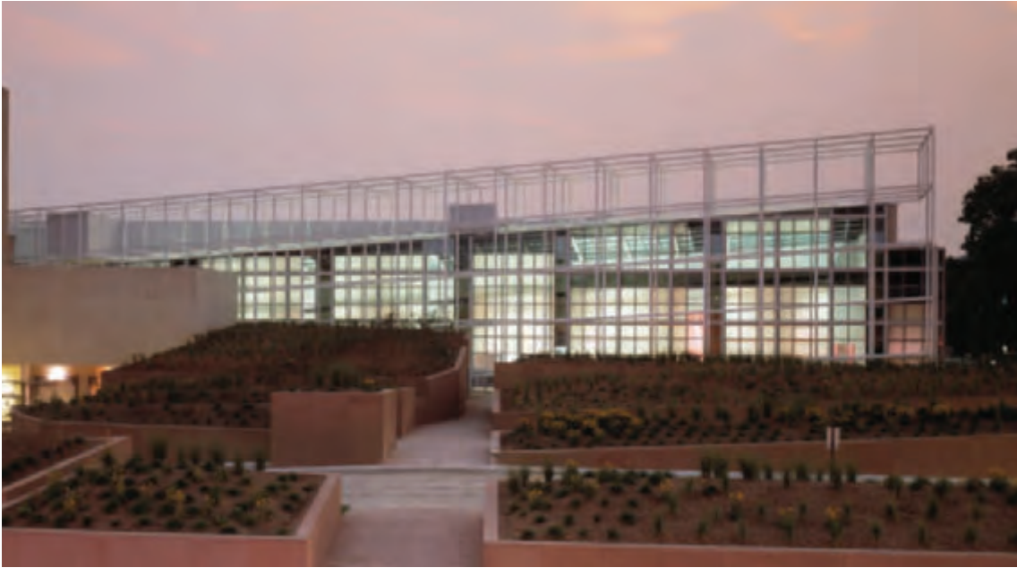
6. The scaffolding grid emerging to the rear of the building where its raked form is clearly visible.
