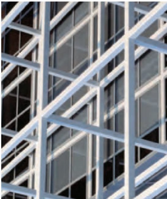
14. Detail of the end of the scaffolding grid which marks the public route across the site.
