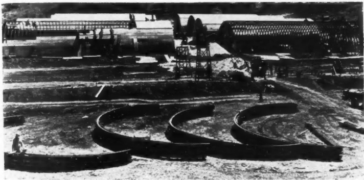
Stran Steel arches ready for use for warehouses in the South Pacific. Note building ready for covering. Official U. S. Navy Photograph.
