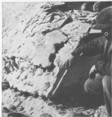
CONCRETE CRACKS under 150 ton lift.
