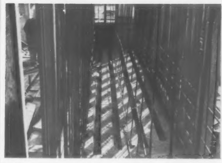
7, grooves formed in the walls of the cyclotron chamber to provide a key for radiation protection between each pour of concrete.
