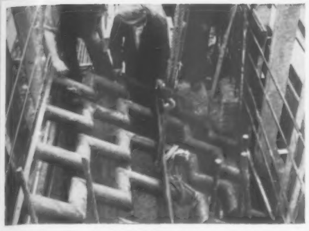
6, air inlet ducts of the cyclotron chamber being manoeuvred into position. Ducts are staggered for radiation protection.
