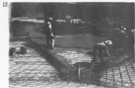
maximum tensional loading occurs at the centre of each straight side. The concreting of a similar slab is seen in 12, its
